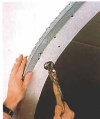
Nail bottom leg first. With the cut leg facing upward, the author presses the bottom leg tight against the drywall before nailing.
