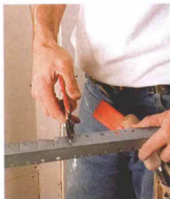
The old-fashioned way. As with \frac{1}{2} -in. drywall, a series of cuts on one side gives metal corner bead the flexibility to follow a curve.
