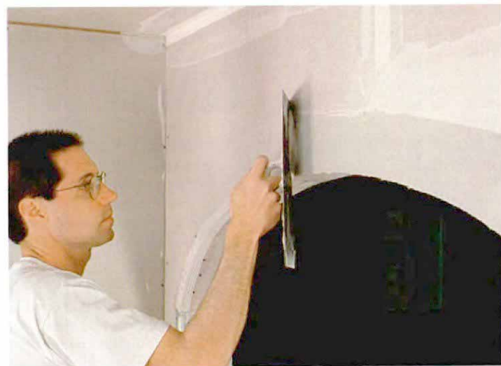
Tape and finish are applied the same way they are for regular corner bead. After taping the joints in the drywall, the author applies a heavy coat of joint compound with a 6-in. knife, then feathers it out with a 14-in. trowel.
